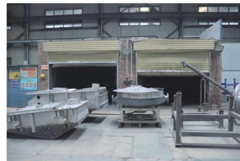
喷砂房 Sandblasting room
